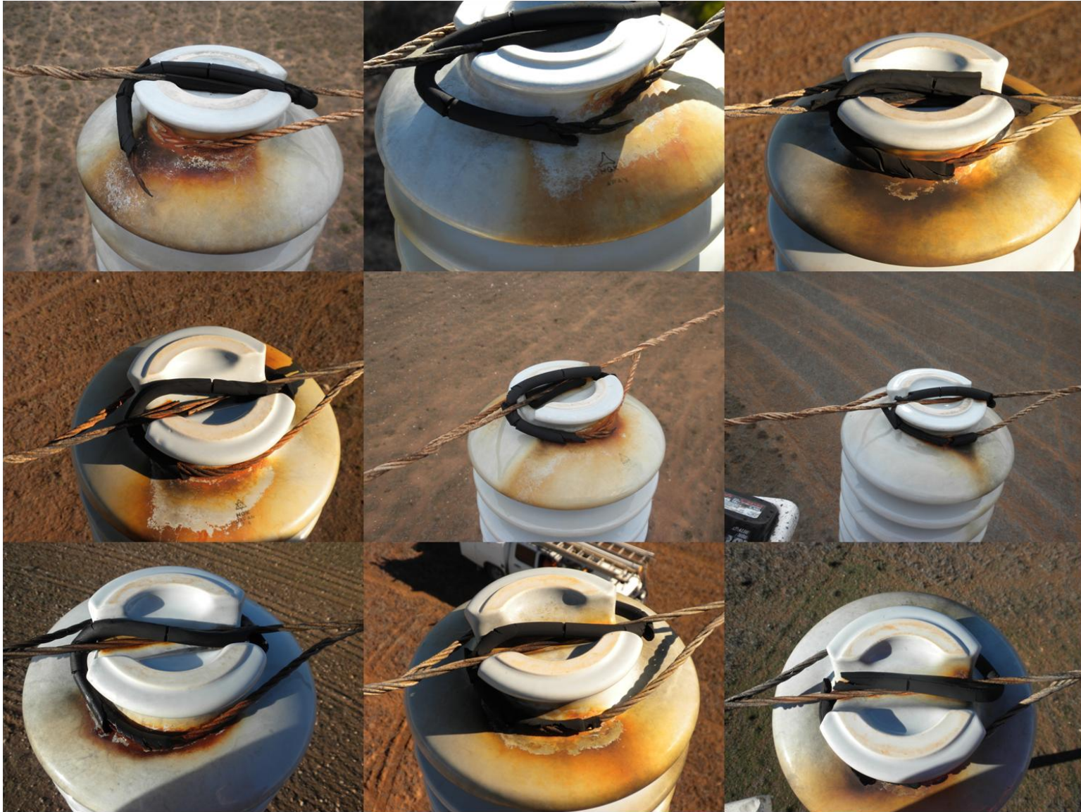
Figure 27: Examples of issues identified
